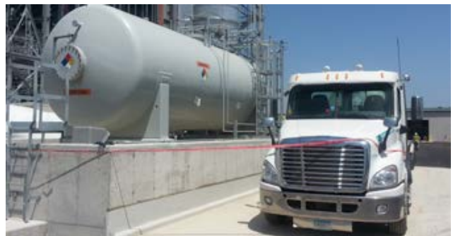
High-visibility magnetic level indicator with magnetostrictive transmitter supports the offloading of ammonia at a combined cycle power plant
