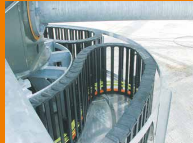
Rotating energy supply system using RBR E4 in a telescope, which is exposed to strong snow and sand.
