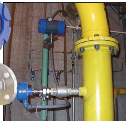
FIGURE 9. A thermal mass flowmeter with remote electronics is used to measure the biogas flow from an anaerobic digester. The probe is located roughly 3 ft from the floor, and the remote head permits the operator to view the display. A retractable probe assembly is used to permit the removal of the probe from the pipe to ease maintenance while minimizing leakage of a combustible gas
