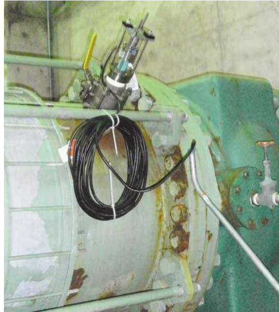
Figure 3: An FPI Mag Flow Meter Installed In A Lift Line
