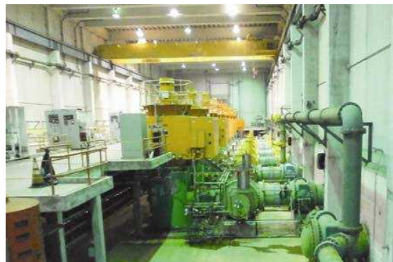
Figure 2: Large Input Feed Lines
