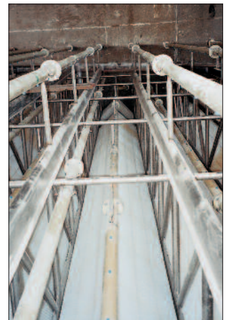
LTV 110, view from the top, in a flue-gas desulphurization plant
