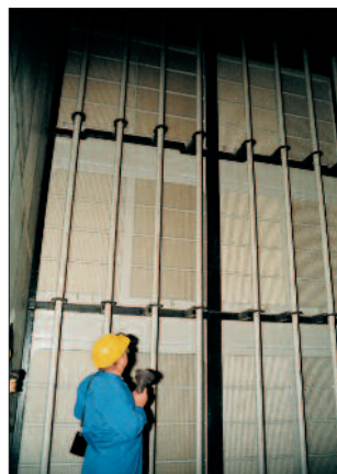
Installed LTH 100 in a flue-gas desulphurization plant
