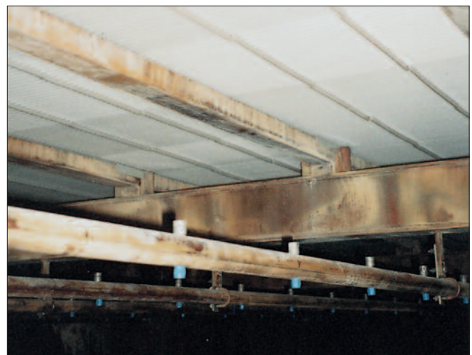
Installed LTV 400 in a flue-gas desulphurization plant
