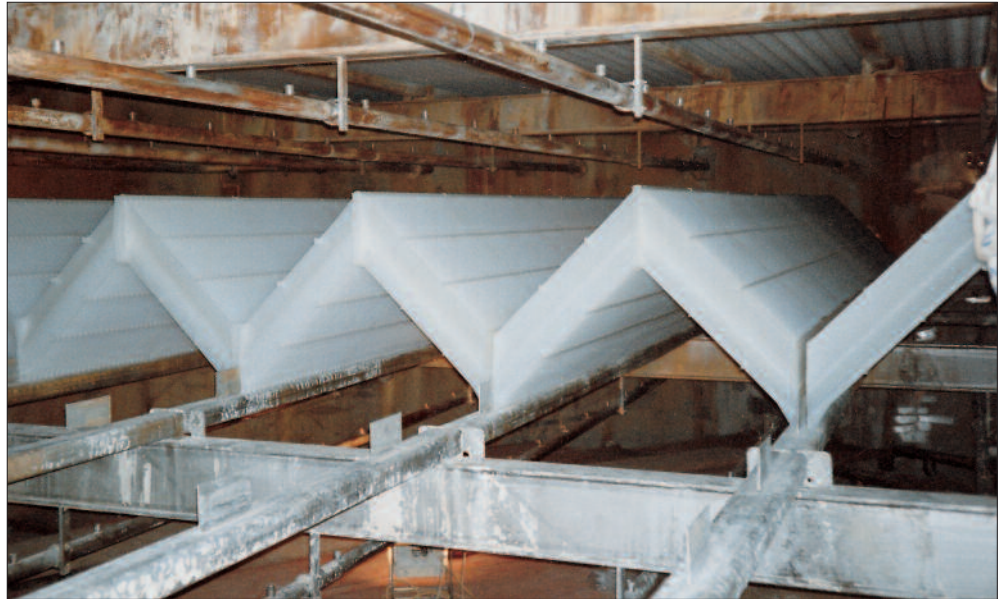
LTV 110.33.-B in a wash tower
