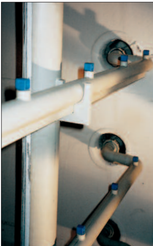
Detail nozzle spray system
